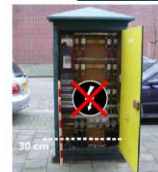
Transformer houses are frequently submerged
