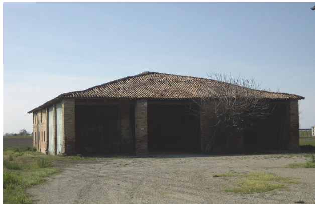
Stalla (foto post-sisma)
