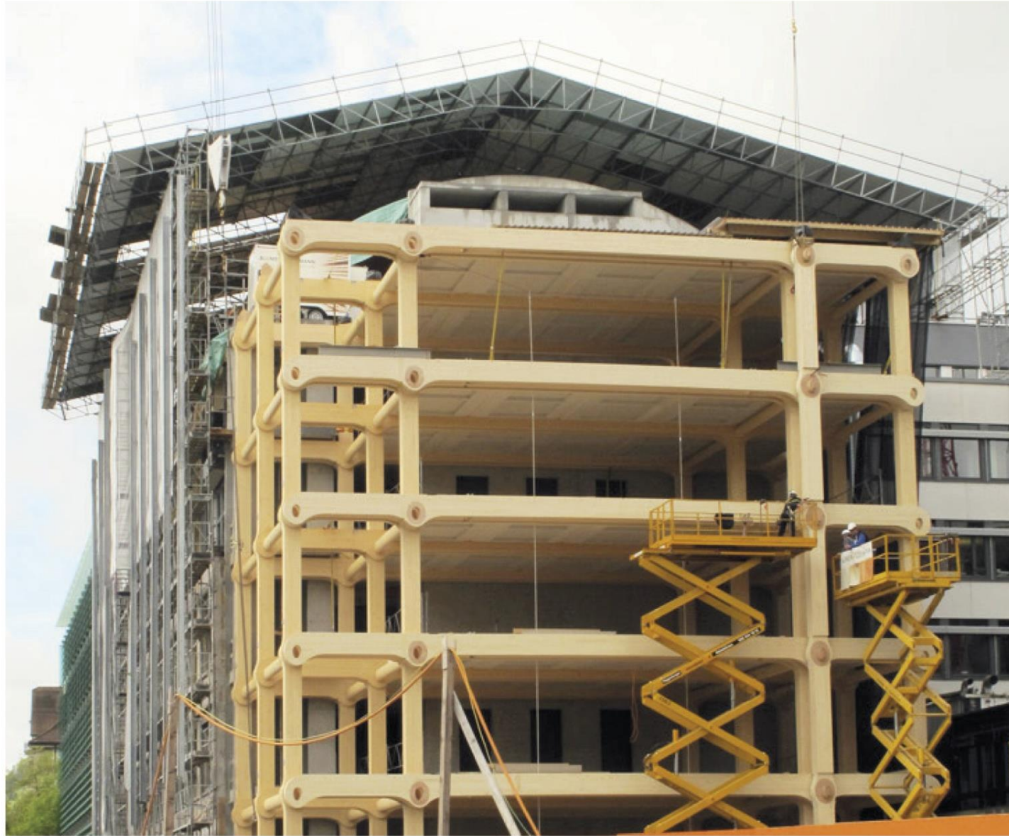
The structure of the Tamedia Office Building, in Zurich, is realized with 2000 m 3 of wood.
